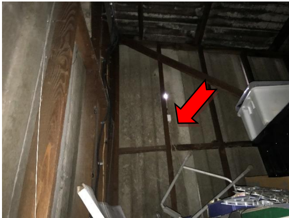
Photo 3. Interior, roof space, wall and ceiling – suspected non-friable asbestos-containing corrugated fibre cement sheeting
