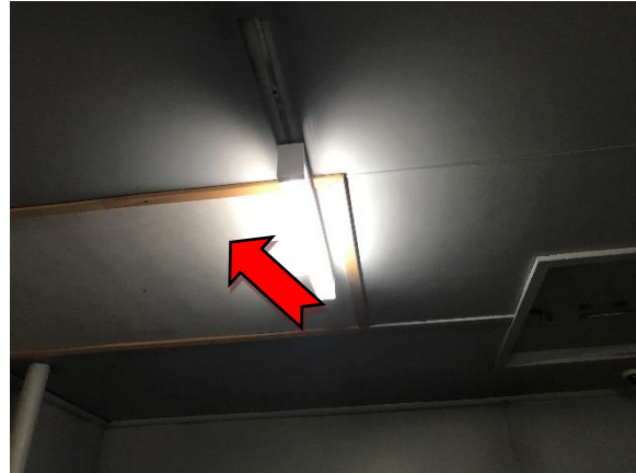
Photo 2. Interior, store room 1, ceiling – non-friable asbestos-containing fibre cement sheeting
