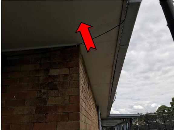
Photo 1. Exterior, throughout, eaves – non-friable asbestos-containing fibre cement sheeting.
