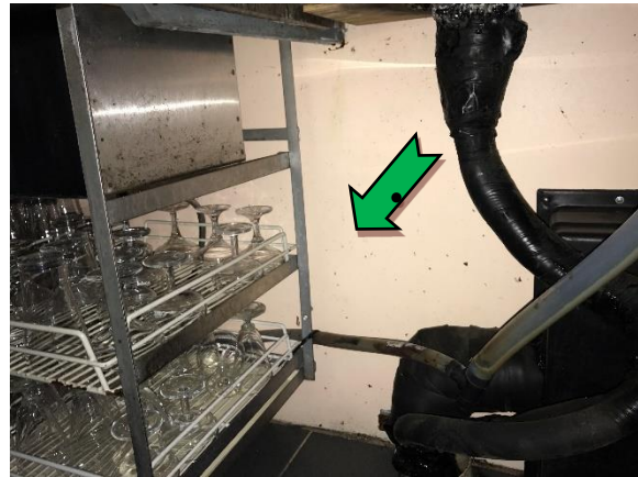
Photo 4. Interior, main club room, beneath bar, infill panel – non asbestos-containing fibre cement sheeting
