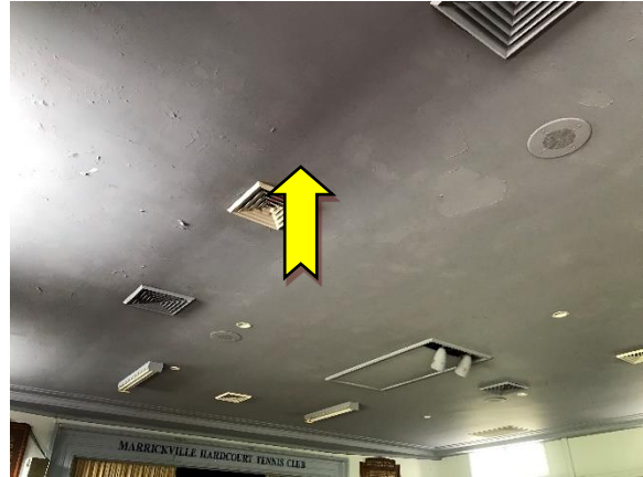
Photo 8. Interior, throughout. Ceiling - suspected lead-containing white upper paint system.
