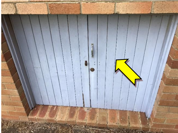
Photo 7. Exterior, south elevation, doors - suspected lead-containing blue upper paint system.
